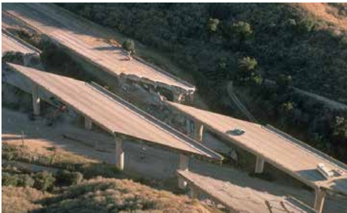
Aerial view of Interstate 5 collapse at Gavin Canyon in Los Angeles County, January 1994.
