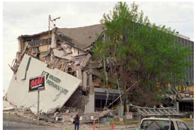
The Kaiser Permanente Building after the Northridge Earthquake. Photo taken on Saturday, January 22, 1994 by Gary B. Edstrom.
