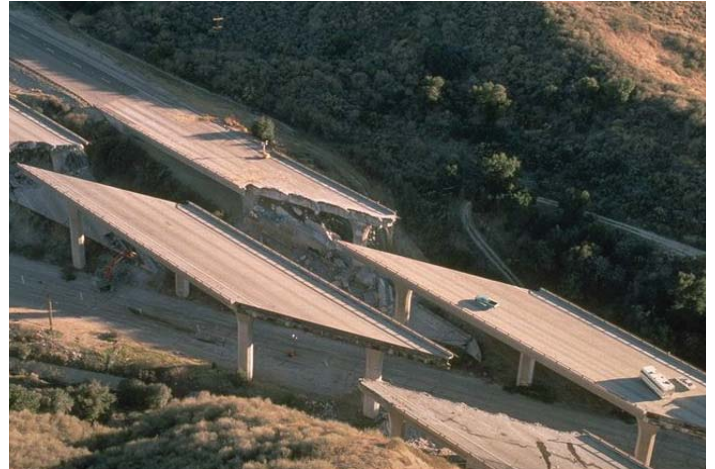
Aerial view of Interstate 5 collapse at Gavin Canyon in Los Angeles County, January 1994.
